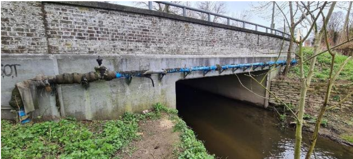
Figure 12: View of the A23 Brighton Road bridge over the River Mole from the North
